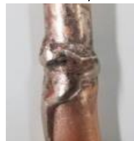
Poor Quality Joint
