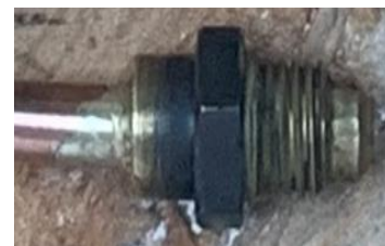
Copper to brass brazed joint
